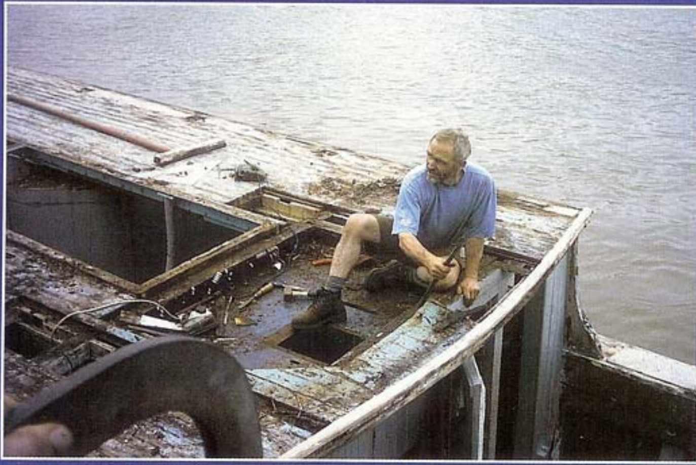
Repairing the wheelhouse floor. There was much timber replacement required throughout the whole vessel.
